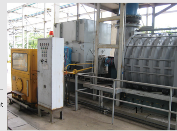
粤电湛江奥里油电厂 Zhanjiang Aoliyou Power Plant
